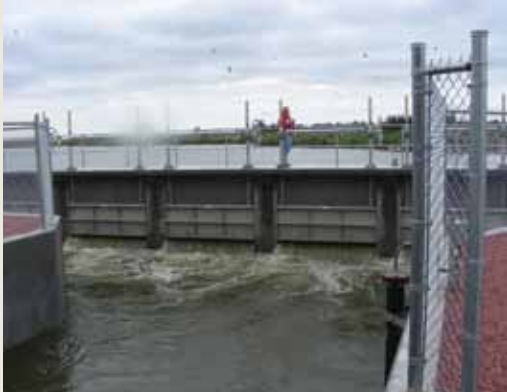
Pat Grant walks across the newly completed Taylor-Ord canal head gate near Taylor. The head gate had to be built to replace one that was washed-out by floodwaters in 2010.
